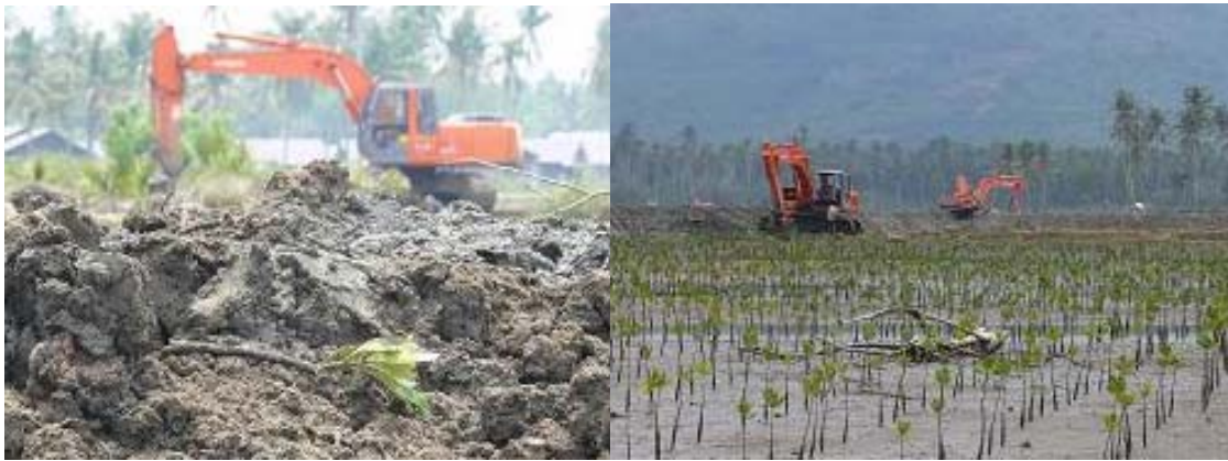
Figure 4-10. Construction of ditches (pond rehabilitation) has damaged the mangrove already planted (Lham Ujong village, Aceh Besar)
