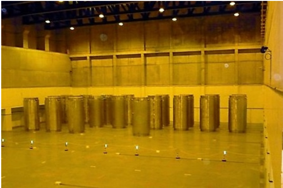
Image of the Individualised Temporary Storage at the Trillo nuclear power plant.
