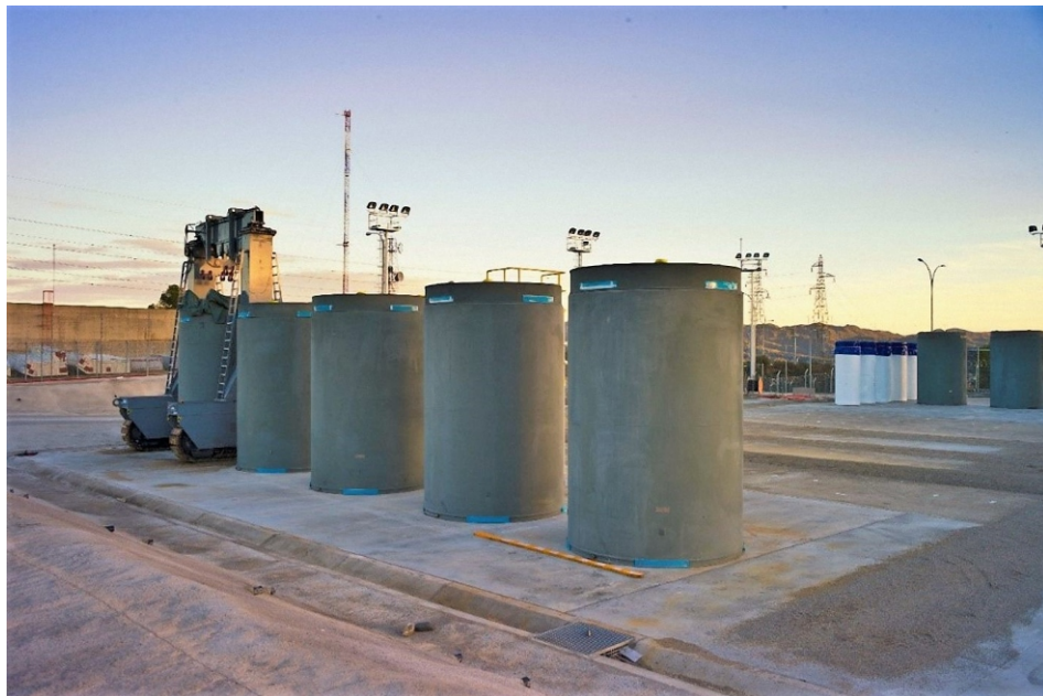
Image of the Individualised Temporary Storage at the Ascó nuclear power plant.
