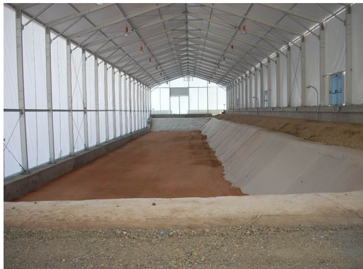
Interior of the VLLW cell at ENRESA's El Cabril disposal facility.
