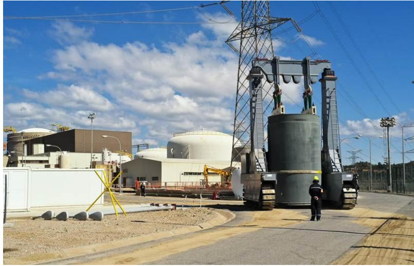
Transport of spent fuel cask to the Ascó nuclear power plant ITS facility.
