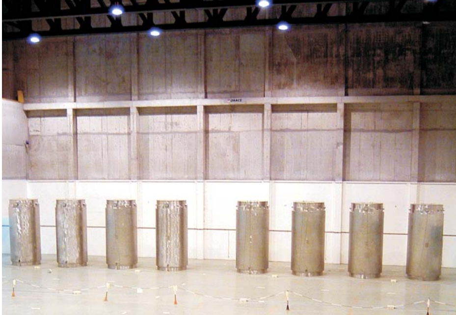
Spent fuel management facility: temporary storage at Trillo NPP.
